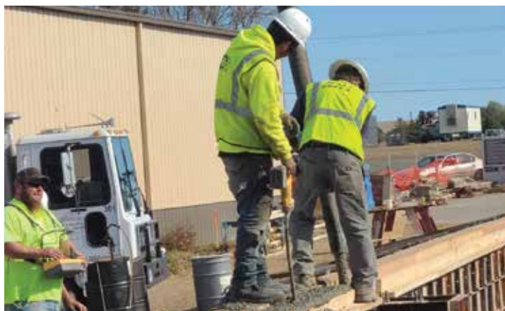
From concrete workers and bricklayers to framers, carpenters, HVAC experts, electrical professionals, plumbers, window installers, roofers and more, well over 100 tradespeople will have contributed their expertise to making our reconstructed hospital a reality.
