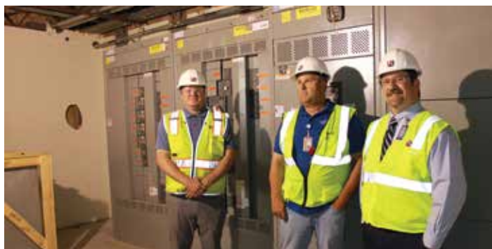
The switchgear is the electrical power system that runs the hospital. It's the brains of our 30-circuit electrical system. It took 22 long months for our new switchgear to arrive, but it's finally here, and we're now getting the entire electrical system updated and switched over.
