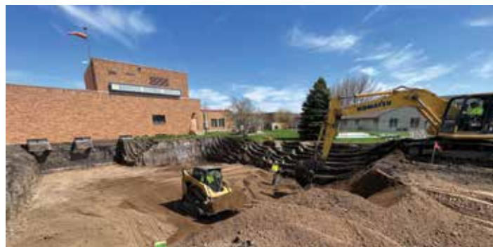
A new ambulance garage is being built next to the new addition.
